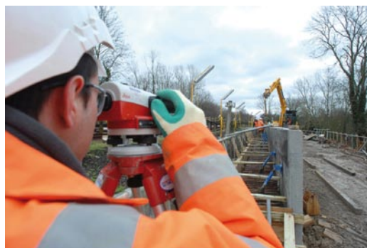
ABOVE Metronet civils projects and maintenance are now being completed under an NEC framework (courtesy Metronet Rail)
