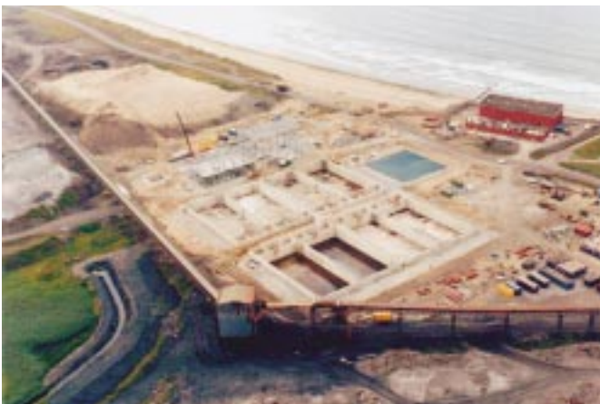
The £30 million Afan project has set a new benchmark for partnering agreements
